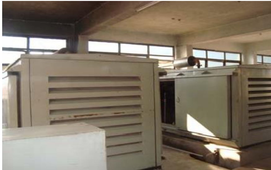
POWER HOUSE AND GENERATION UNIT
